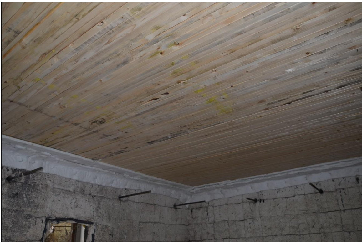
Figure B-4. Inside of Furnace prior to Testing.
