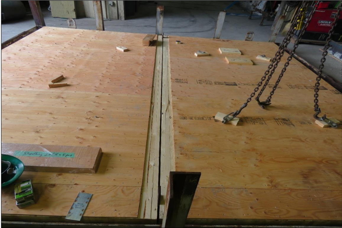
Figure B-1. DLT Panels with Plywood Sheath Nailed and Put in Place with 1/2-in. Gap.
